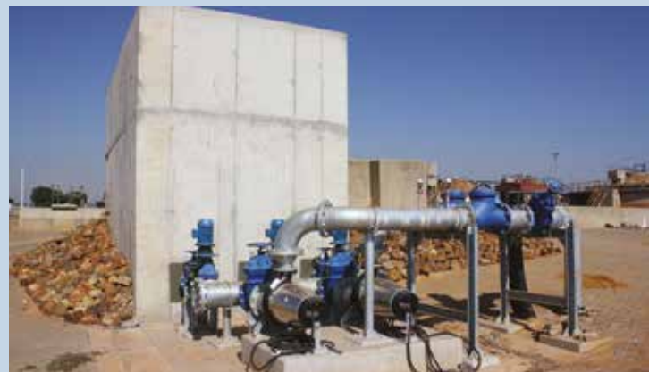
THE NERADA PLANT IN HARTEBEESTFONTEIN WATER CARE WORKS
